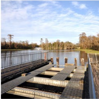
Pre-existing weir with failing maintenance deck
